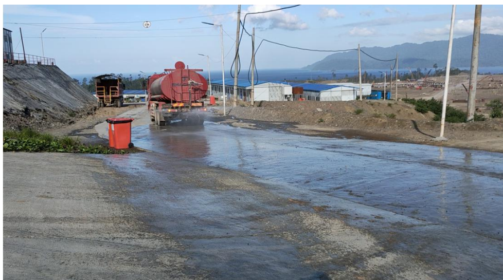
Sprinkler at site
